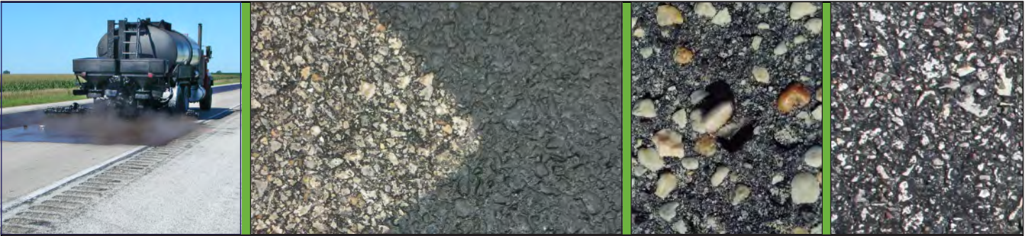
GSB-88 significantly postpones water damage to milled-in grooves without compromise to pavement design.
